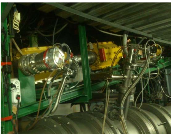
Figure 4.2 LU-20 injection + place for rotary magnet
