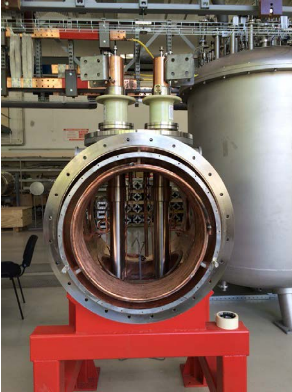
Fig. 20. Current leads cryostat
